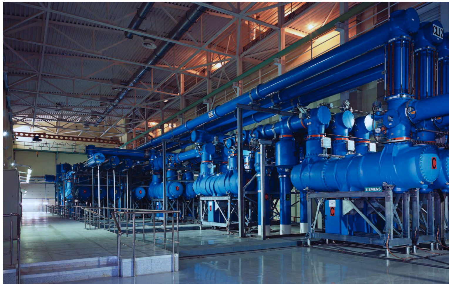
Gas-insulated switchgear (GIS) for 500 kV in Beskudnikovo substation. GIS installed by Siemens is a key element in the historic modernization effort.
